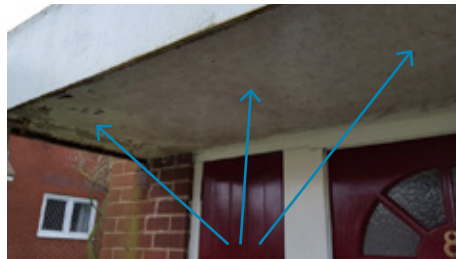
More insulating board made using asbestos
