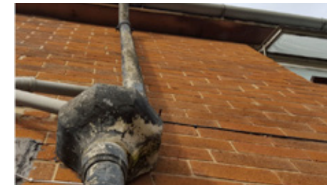
A cement downpipe made with 10-15% asbestos
