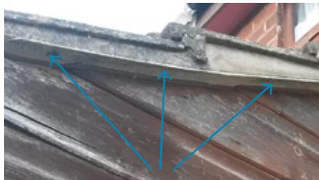
Insulating board made using asbestos
